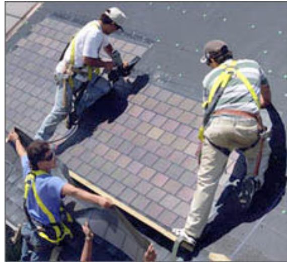
PV roof shingles
